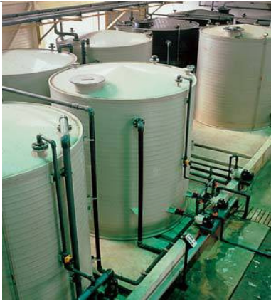
PP STORAGE TANK
