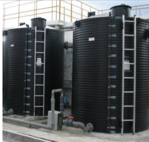
HDPE ACID STORAGE TANK
